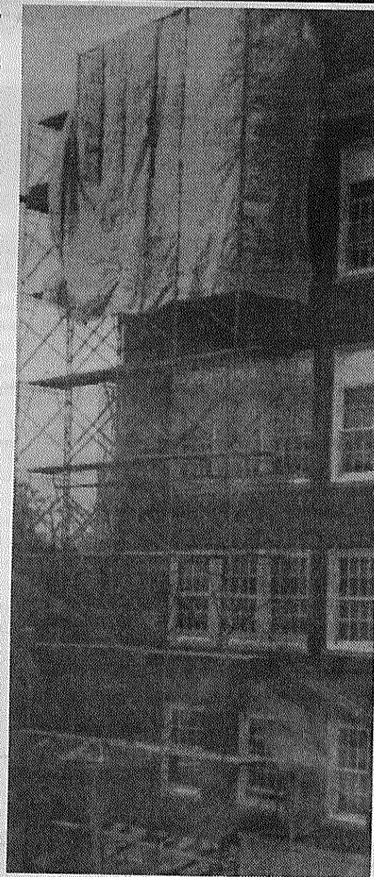
SHS in the process of repairs after wind damage. Photo by Goldschmidt
